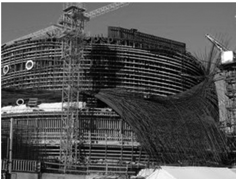
Figure 1: Collapsed reinforcing rods in the containment of Leningrad NPP No. 2, unit No. 1.
